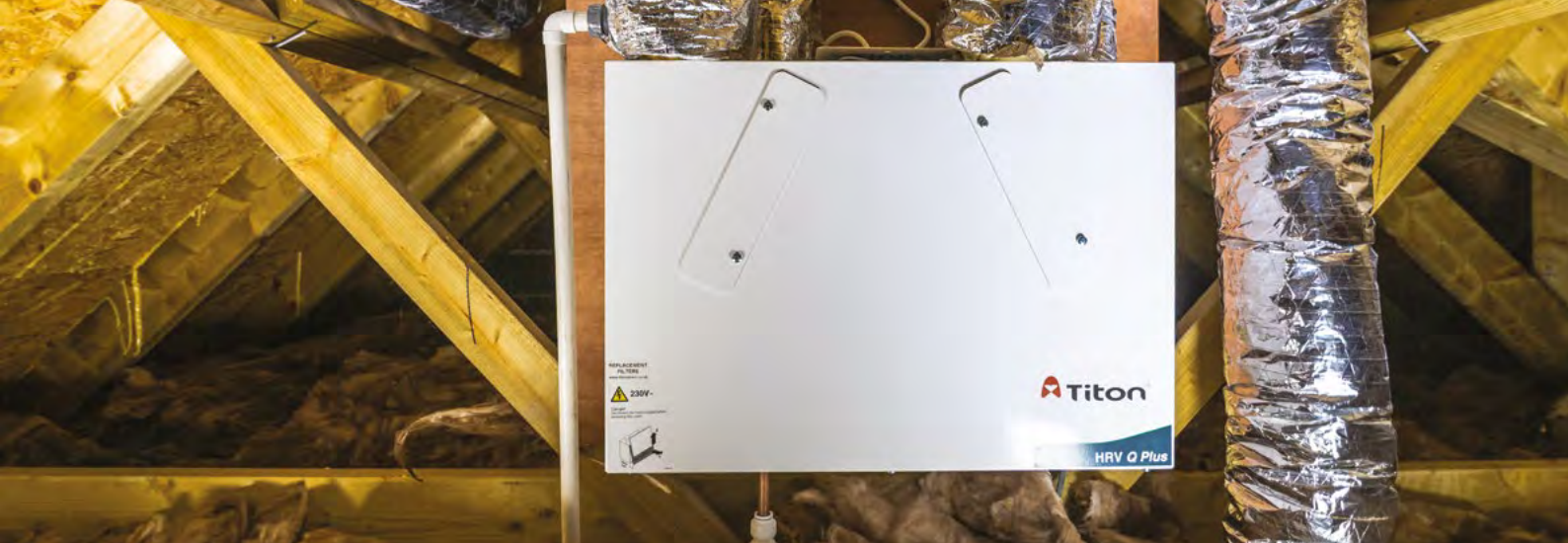
One of our HRV units in-situ
